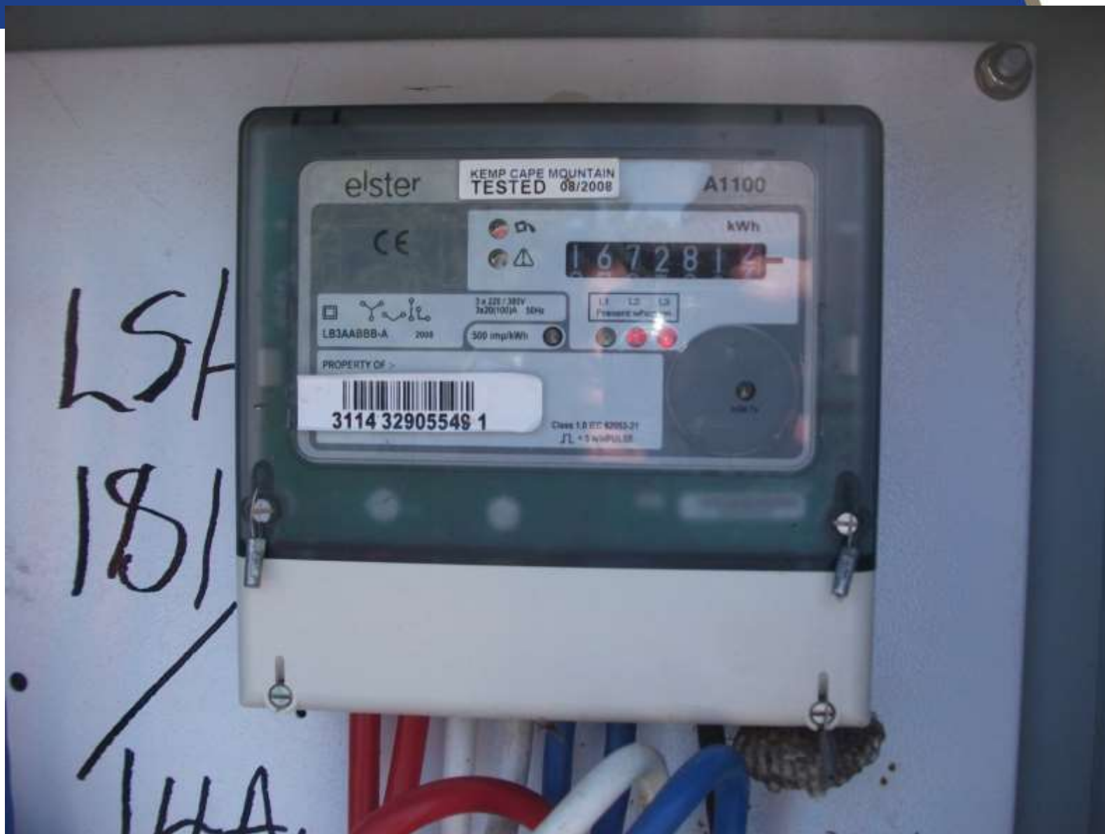
Phase wires cut
